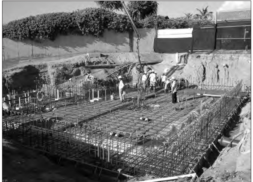
Preparations are made to pour concrete for the foundation of the Education Center in May. • Photo by Riecke Sunnland Kono Architects Ltd.
