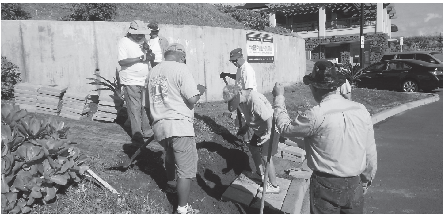
Lions Club members on Aug. 26, 2017, installed a 40-foot concrete brick walkway at Maui's Nisei Veterans Memorial Center.
